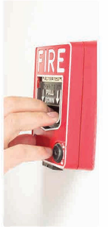
Fire Fighting Systems
