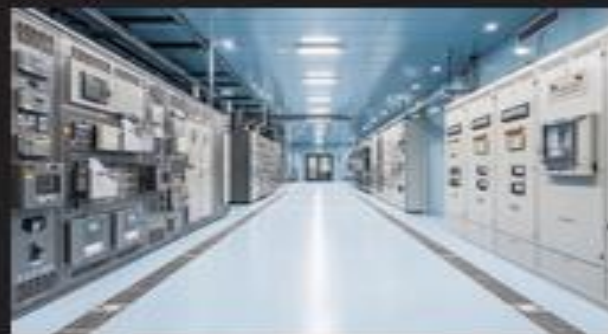
Emergency Power Backup
