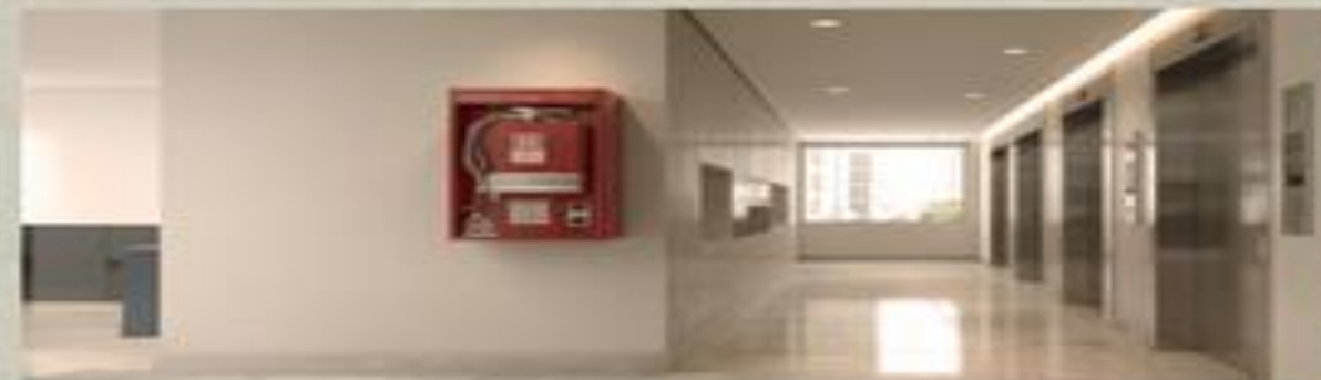
Fire Detection & Control Systems
